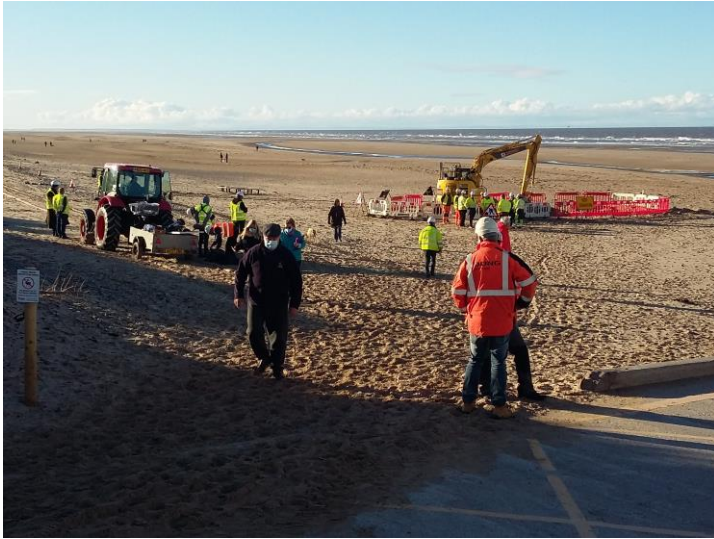
Sunday's operations as the laying vessel carrying the cable neared the beach.
